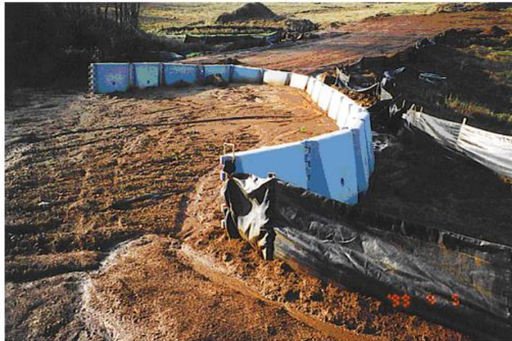
Figure 24 (g) Pre-fabricated barrier
